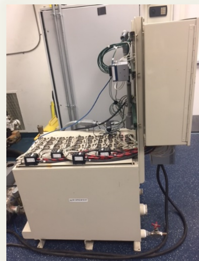
250kW Resistive Load Bank
