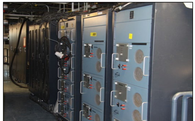
Cell, Module & Battery Cycling Equipment
