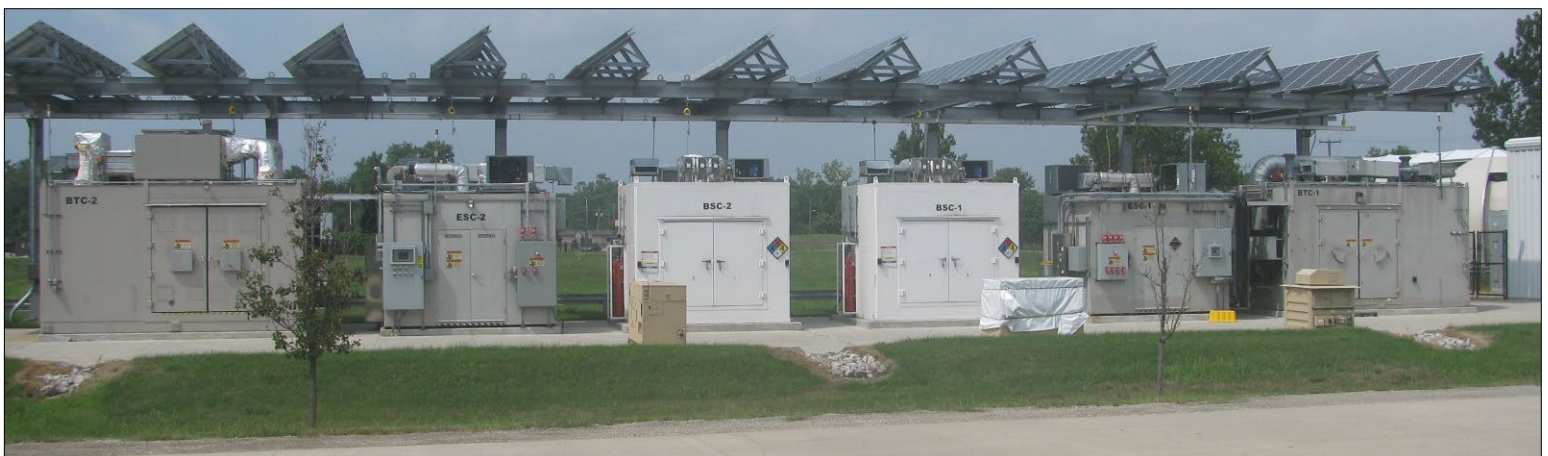
Outdoor Pack Test Chambers
