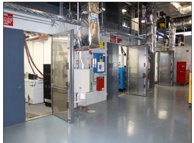
Internal Cell/Module Test Rooms
