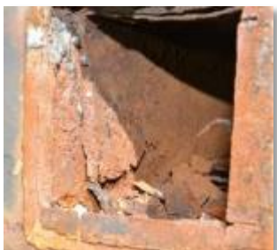
Frame member affected by severe in-service corrosion
