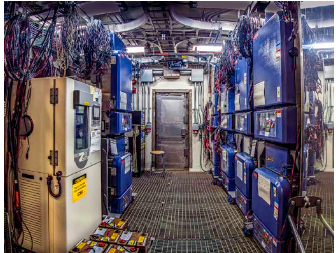
Internal Cell/Module Test Room
