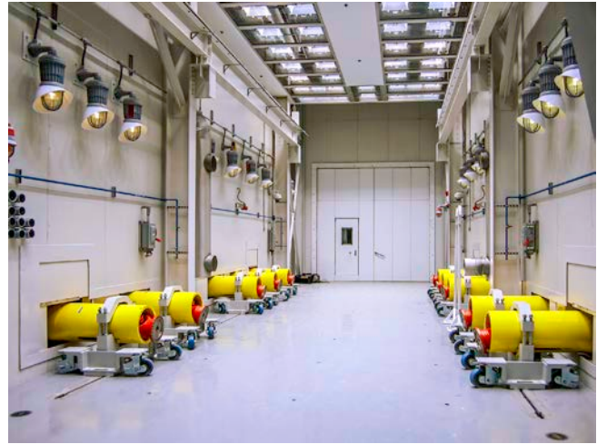
PEVEL - Test Cell Interior
