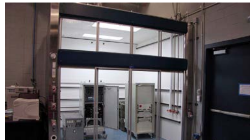
Large Walk-In Fume Hood
