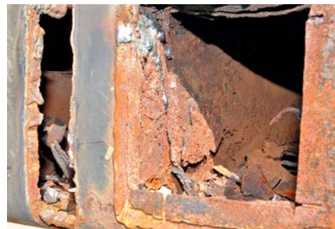
Frame member affected by severe in-service corrosion
